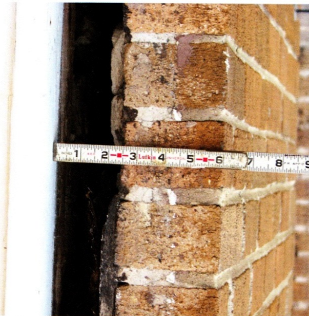
Displacement of veneer in excess of two inches.
