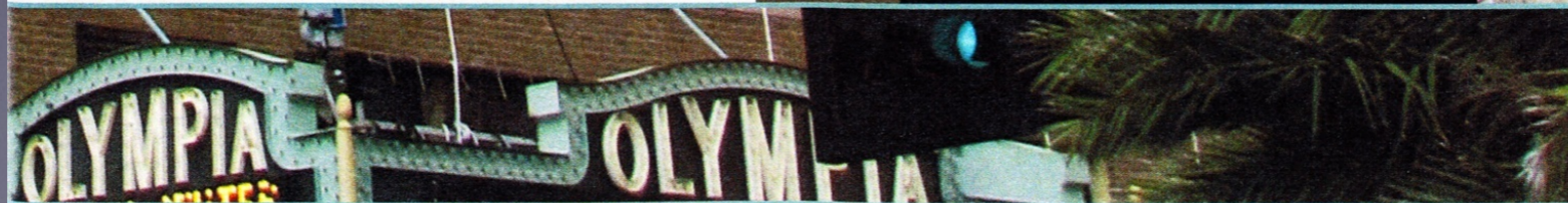
Restoration specialists encountered severe cracks and façade deterioration around the corners of the Olympia Theatre.
