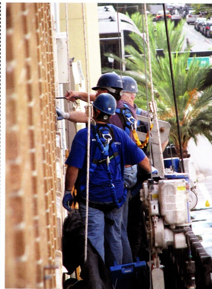
Helifix on-site quality control support team and STRUCTURAL'S specialty repair contractors perform installation.
