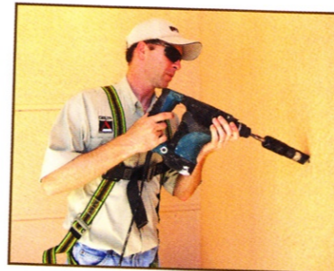
The ties were installed at a 45-degree downward angle to increase the surface area of the helical tie embedded in the stucco, increasing the pull-out capacity of the pin from the stucco.
